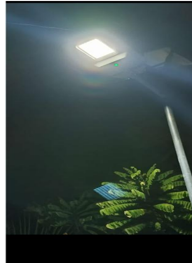
Fig 2. 300 W Solar LED Street Lighting System
